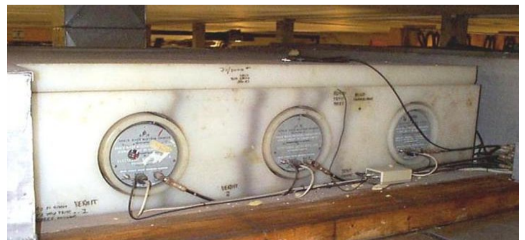
Tubes of the neutron monitor located in the hangar at SANAE-IV.
